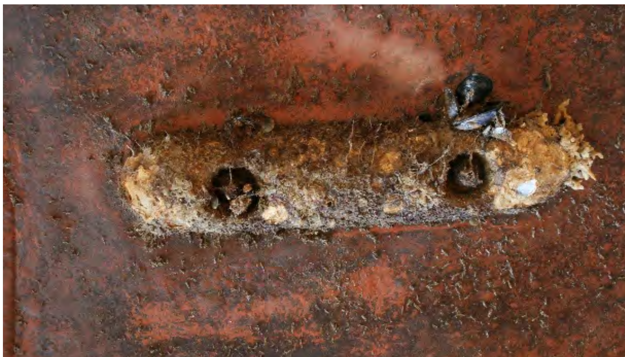
Figure A12 Niche areas: Cathodic protection anode. Source: D. Smith.
